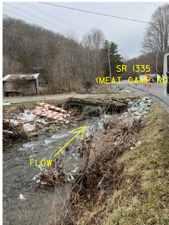
PHOTO #2: VIEW FACING SOUTHEAST UPSTREAM OF DAMAGED BRIDGE NO. 187.
