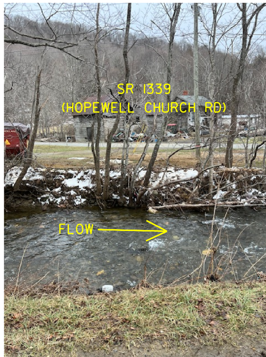
PHOTO #1: VIEW FACING EAST TOWARD END BENT NO. 2 FROM THE VICINITY OF END BENT NO. 1.
